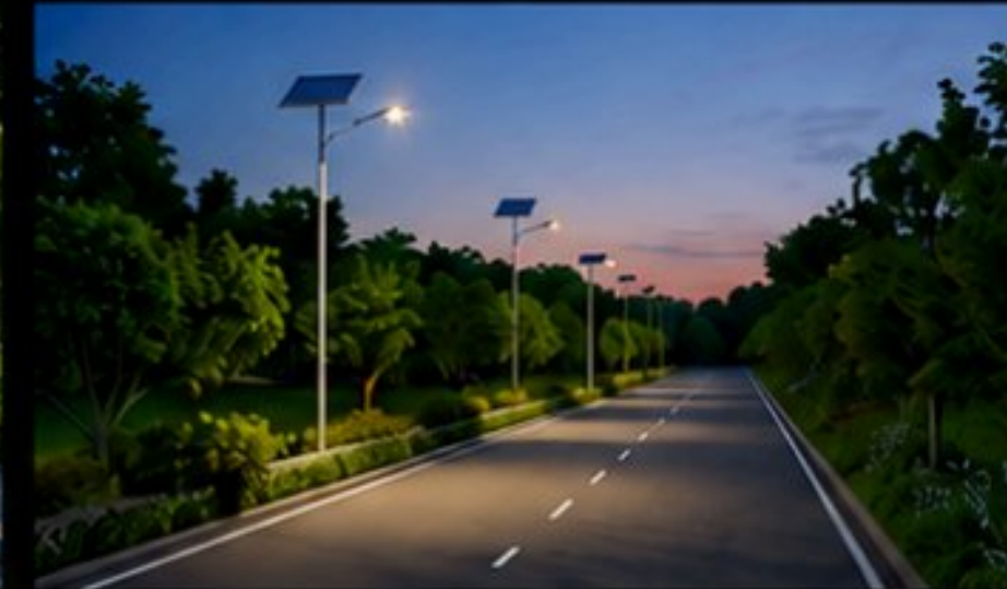
Solar Street Lights
